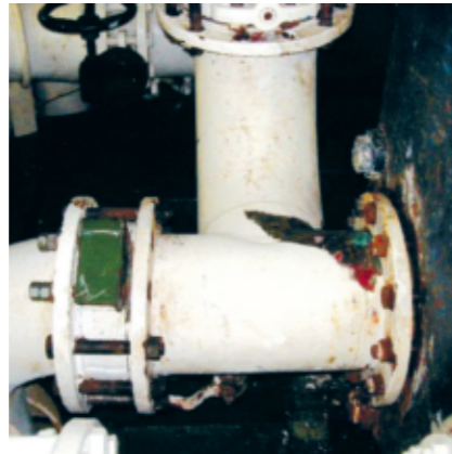
Wrong installation of a copper nickel pipe and titanium plate cooler
