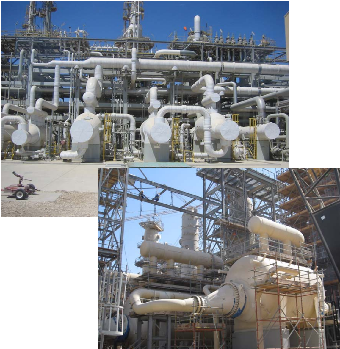
Figure 14. Propane Refrigerant Chillers with GEWA-PB Tubes, LNG Plant Ras Laffan (Qatar).
