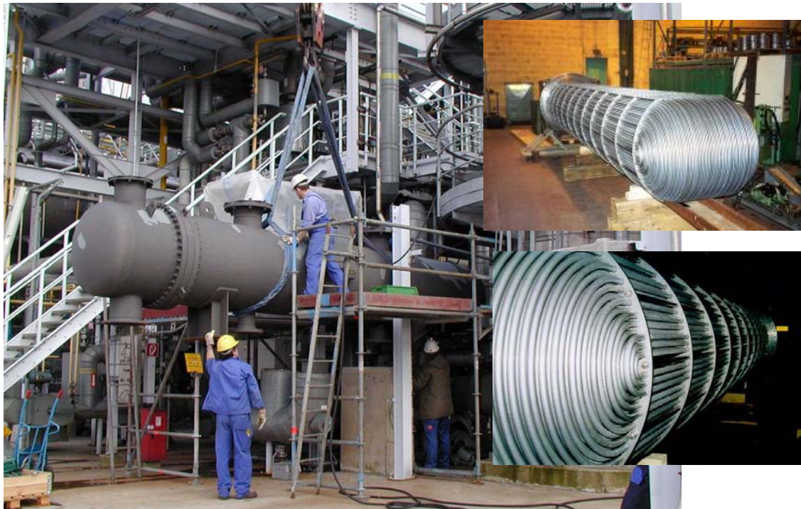
Figure 13. Installation of Horizontal Thermosiphon Reboiler Equipped with GEWA-PB Tubes in a C3 Splitter of a Polypropylene Plant by Lyondell-Basell, Knapsack (D)
